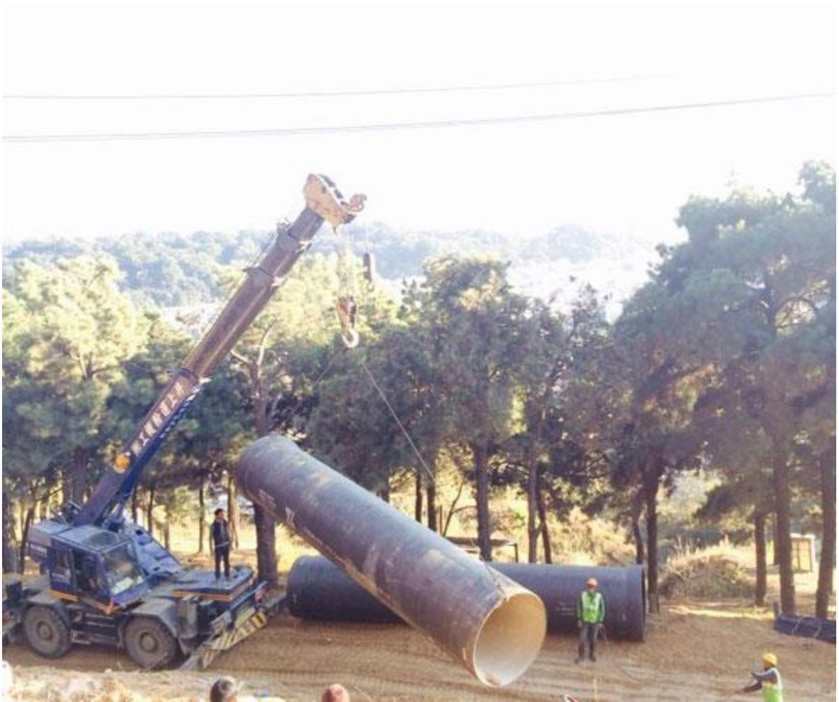
FIGURE 3:- UNLOADING PARTS FROM THE BROKEN TRUCK AND KEEPING IT SAFE PLACE NEARBY.
